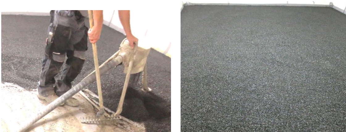
Figure A 2.2: situation during mounting - installation of floor compensating and sound insulating fill
